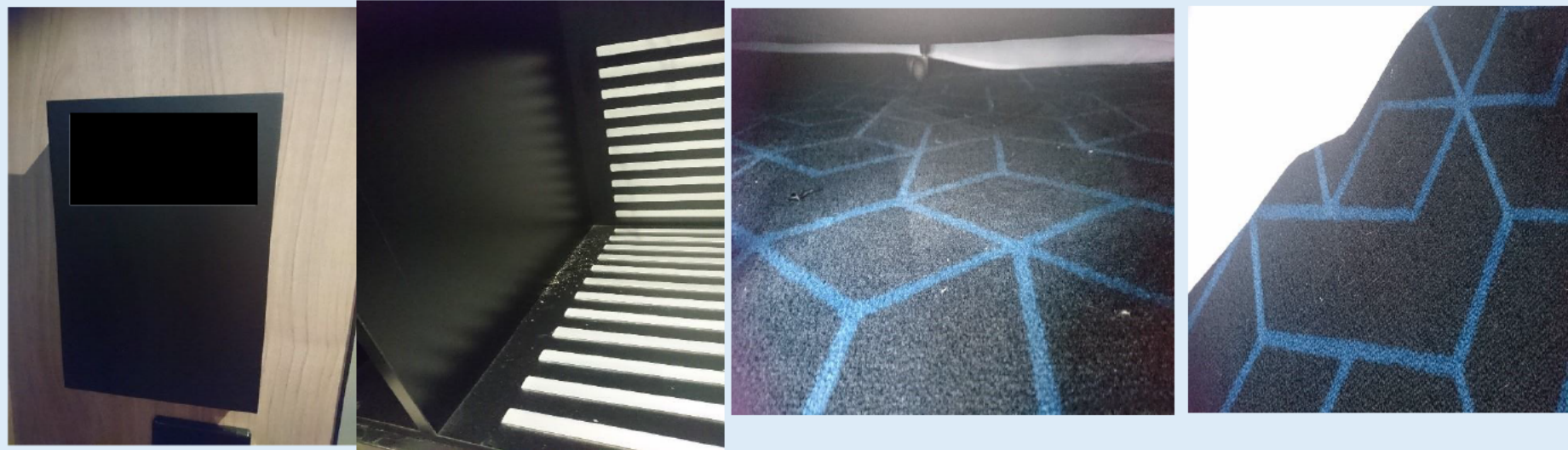
Vacuum under beds not done Properly and touchpoint sanitisation is not done properly
