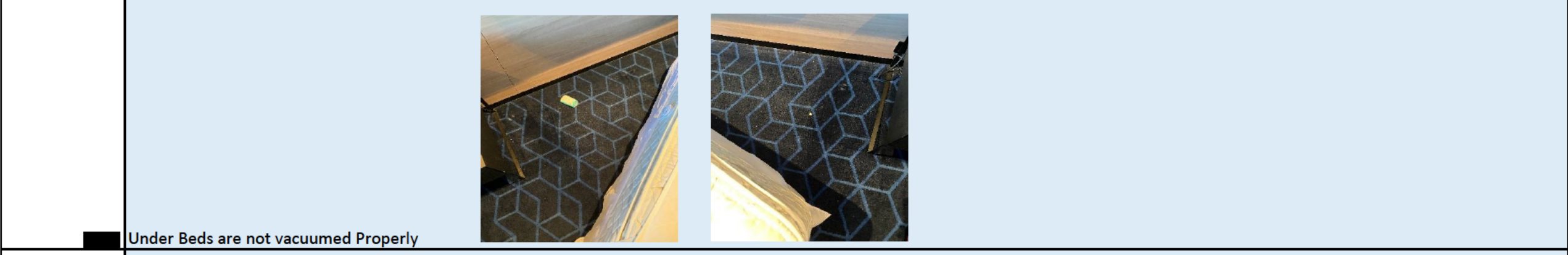
Under Beds are not vacuumed Properly
